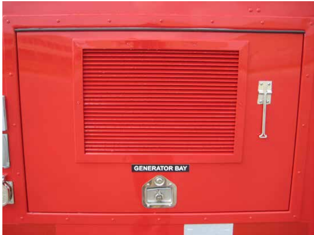
Generator output breaker is behind the removable panel on the generator
