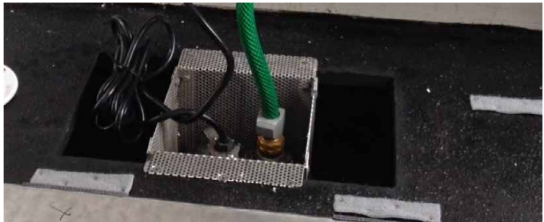
Sump pump assembly in place
