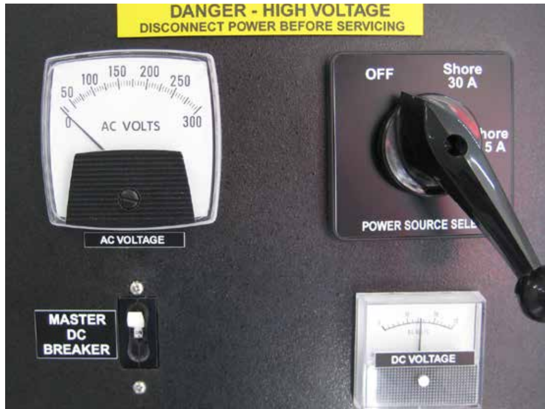
Input Power meter and source selector switch.
