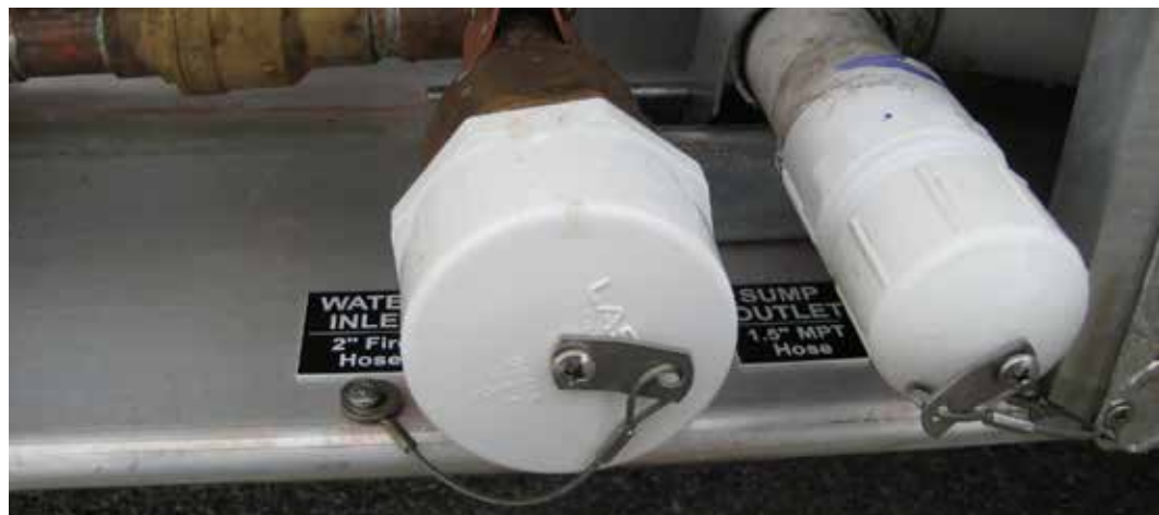
2" input line and 1 1/2" outflow line
