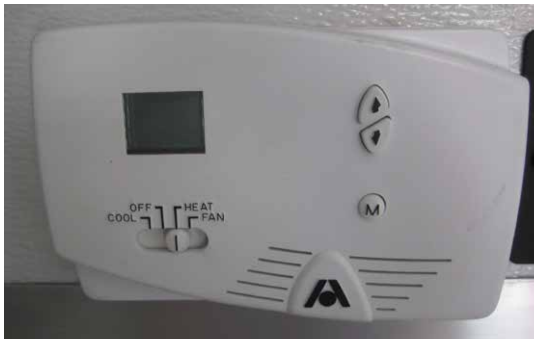
Heater control thermostat.
