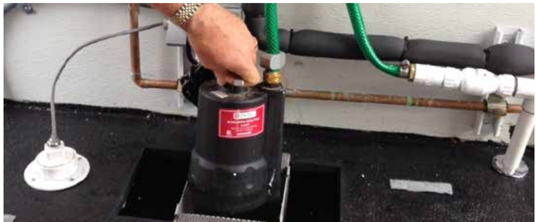
Sump pump just sits in cage for easy removal.
