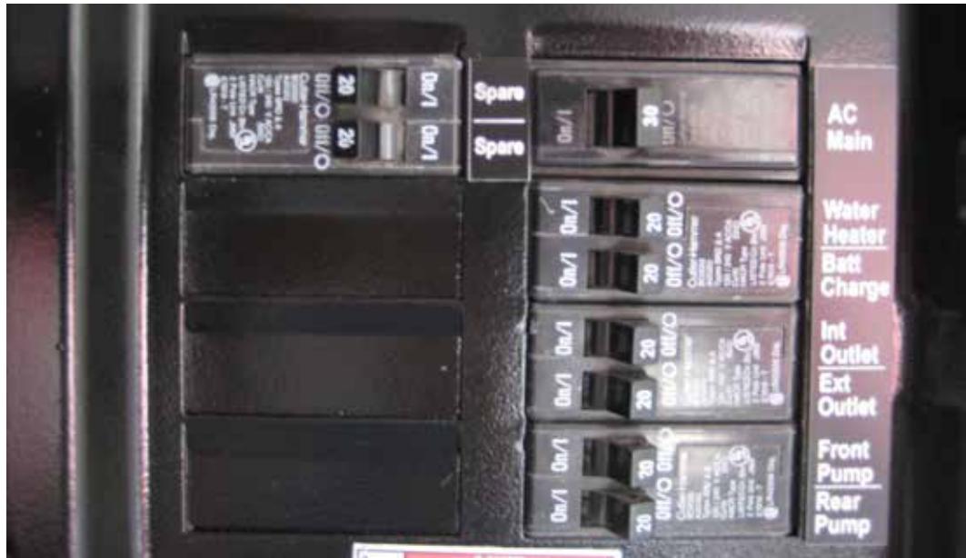
Location of Main AC Breaker.
