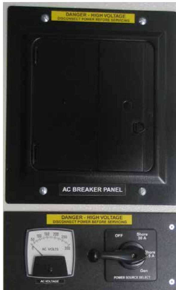
AC breaker panel and source selector switch.
