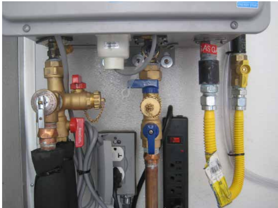
Water and gas valves
