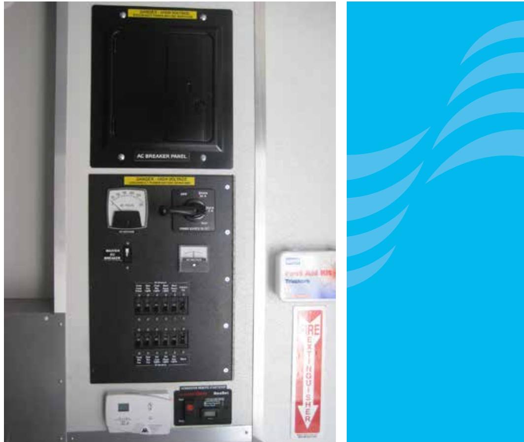
Main AC power panel in the vehicle. AC Main at the top, AC Meter, Source Selector and DC Meter in the middle and DC breakers below.
