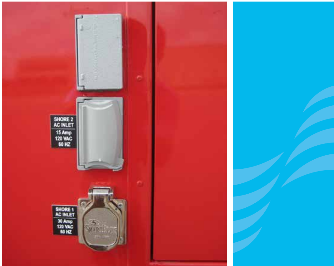
Shore input power connectors on the street side of the trailer.
